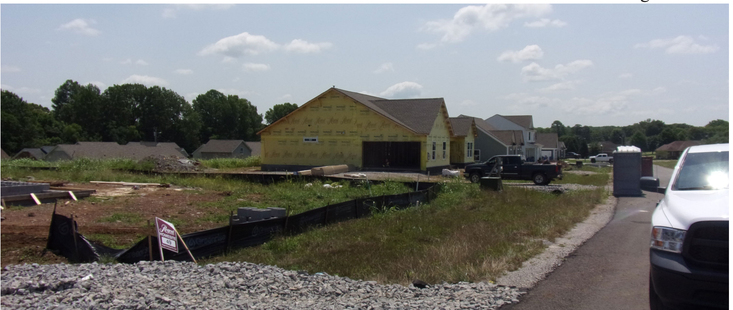
Progress on Sugar Creek Subdivision continues as they work to finish Phase 3.
