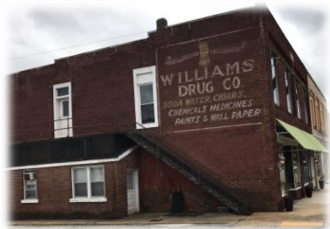
The side elevation of this building faces a significant entry into the Town Square and could be a better architectural element for the area.
