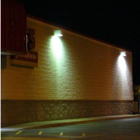
Wall-mounted lighting (fully shielded)
